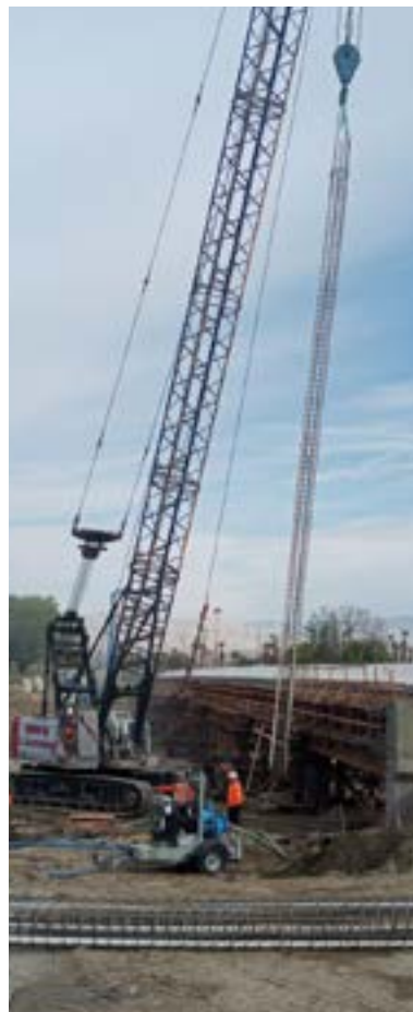
Crews placing the preconstructed rebar cage into the drilled hole with the steel pile, which is then filled with concrete.
