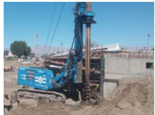
Crews drilling 50 foot holes in the storm channel for the steel piles and concrete.
