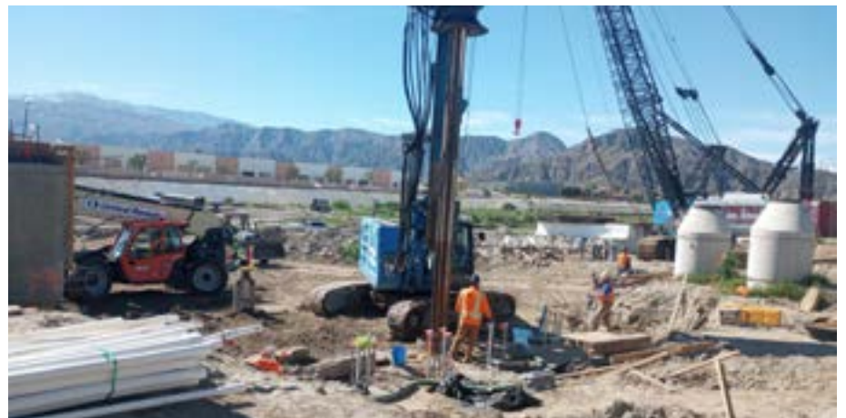
Crews drilling 50-foot holes in the Coachella Valley Storm Water channel for the southbound bridge underground support system.
