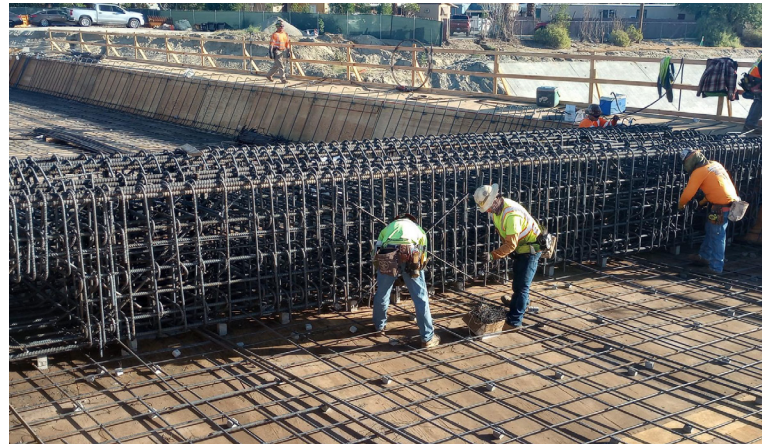
This photo shows crews working on the bridge interior. The stems are the raised rebar as shown in this photo, and the flat area between them is the soffit. Together, they create the bridge interior which will be covered by the bridge deck.
